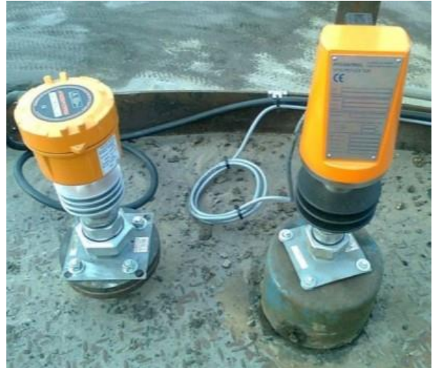
RF Switch and TDR Sensor on top of the tank
